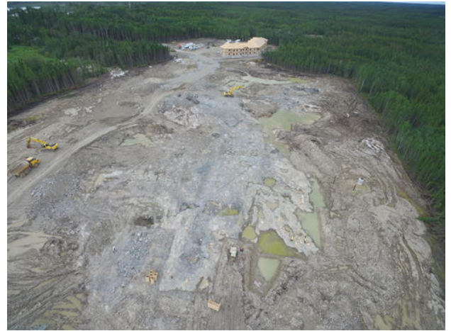
Drone shot of forming labour in area A1 Wayne Dee Jul 17, 2020 3:28 PM
