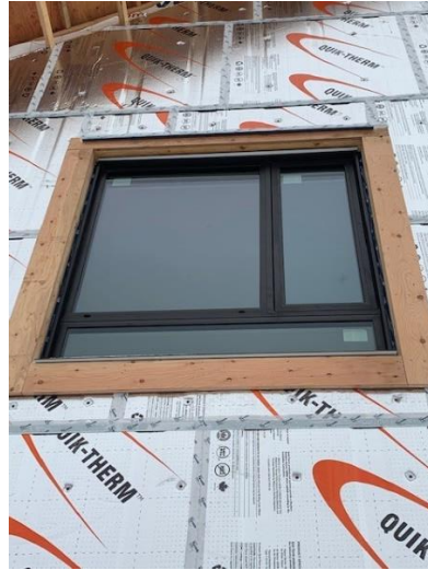
Window Head Flashing Install Upper Level on Gable End – South West Wing
