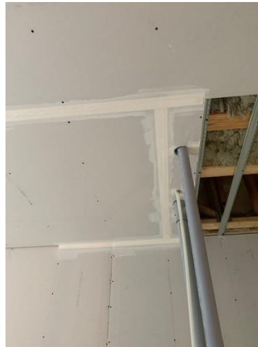
Drywall Tape and Mud Applied to Gypsum Board on Main Floor Ceiling – West Wing
