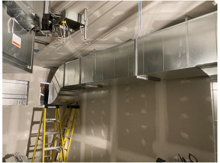
Mechanical Room HVAC Ductwork
