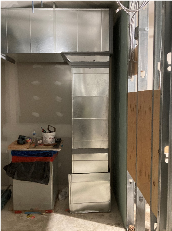
Mechanical Room HVAC Ductwork
