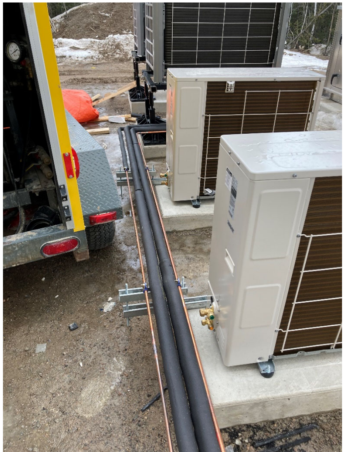
Refrigerant Piping to Heat Pump
