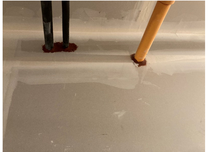
LVL 2 Corridor Mechanical Firestopping
