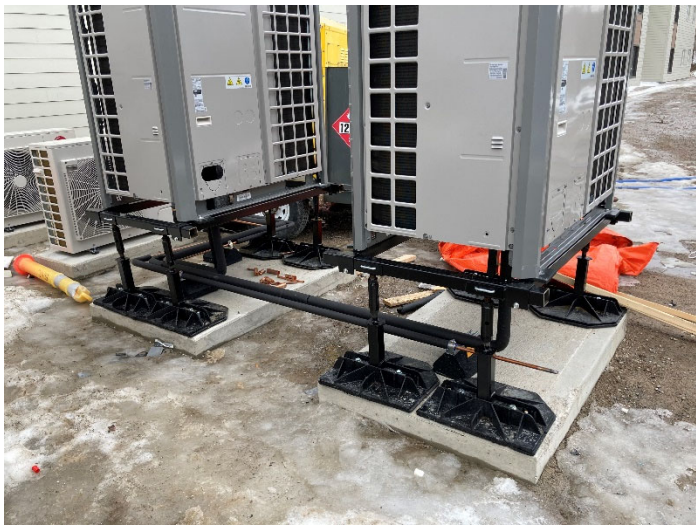
Refrigerant Piping to Heat Pump
